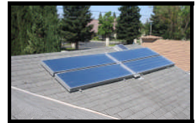
Above: 4: 10-01s = 2 kW system
